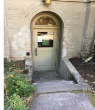
Non-compliant egress point
