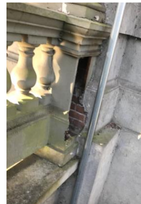
Failing exterior coating I
