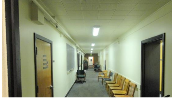
Poor existing conditions
