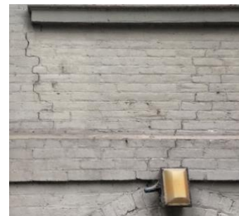
Cracking from window to arched opening
